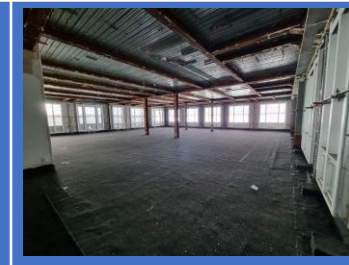
Waterproof protection over live Boots store
